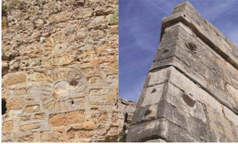
Fig. 14- Left: Acrocorinth ottoman trowel patterns on the masonry (2015), right: Palamidi, relief ottoman symbols, Epameinondas bastion (2018)
