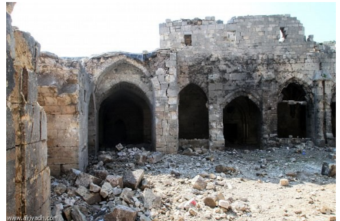
Fig. 12- Damage in the interiors of Crac de Chevalier (Aryad, 2014)
