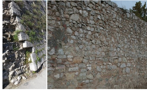
Fig. 13- Building the inner part towards the terreplein (right) and the internal part and scarpa (left) of the Contarini bastion (author)
