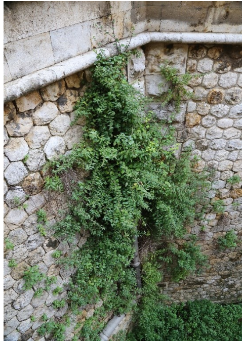
Fig. 4- Nitrophilous casmophytic vegetation ( Parietariion judaicae ) on the wall of Castello fortification realized with exagonal ashlar of limestone
